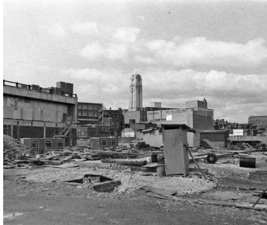
Large areas of the Town Centre were demolished in the late 60s and 70s to make way for the Arndale Centre (Luton Mall).
