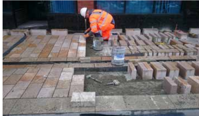
Hull City of Culture 2017 public realm - efficient timetabling and high quality construction work in delivery. The materials and jointing ensured the public realm was accessible and durable for different uses
