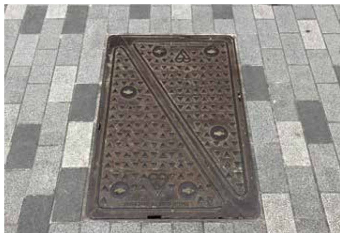
Paving surrounding cast iron covers should be designed to avoid reduce large areas or infill and/or small slivers of paving
