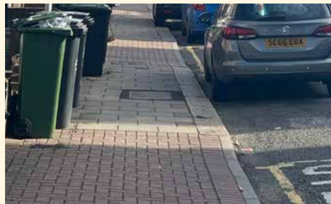
X Inconsistent paving along a streetscape interrupted by driveway crossovers. The changing levels can also awkward to navigate for some users
